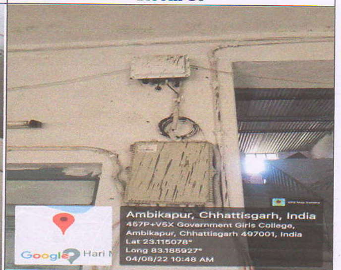
Library Corridor Wi-Fi Enabled
