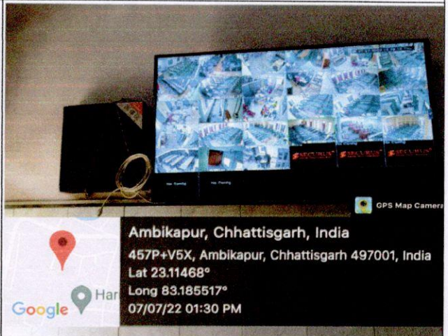
32 PORT CCTV MONITORING DISPLAY & DVR
